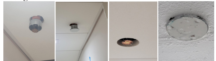
Painted sprinkler cover south side balcony
