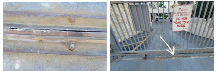
Damaged gate bracket
