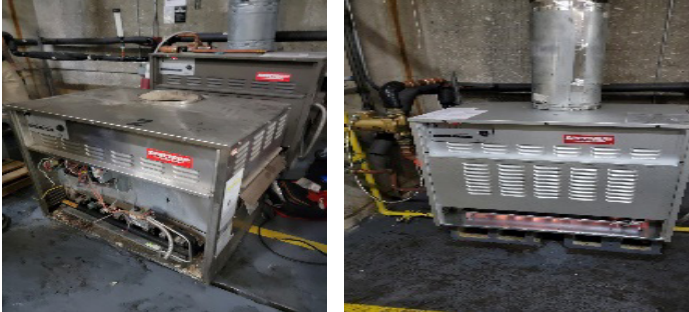
Old boiler heater
