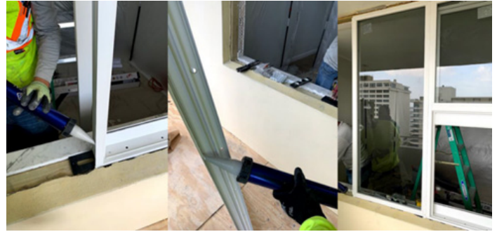
7. Begin installing windows. Dow 795 behind flange where mull bar and wood buck meet window frame.
