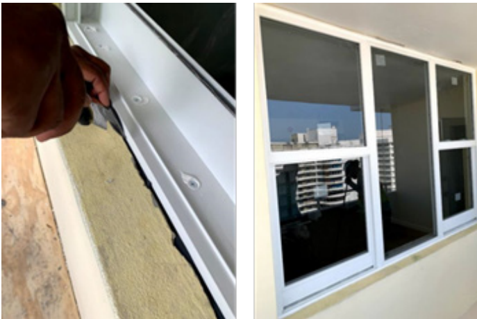
9. Install backer rod where necessary around exterior of window. Caulk entire perimeter with Sika 15LM and metal to metal with Dow 795
