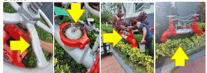
Backflow pump (before)
