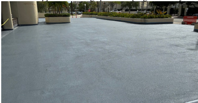
South Contractor Parking - Waterproofing and traffic coatings have been applied. Parking spaces striping underway.
