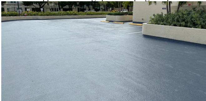
East Visitor Parking - Waterproofing and traffic coatings have been applied. Parking spaces striping underway.
