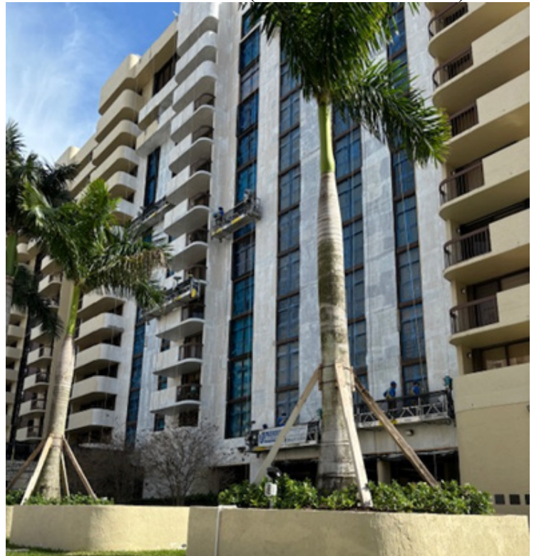
Building NW Corner (Biltmore Way side) – Work started on the front of the building 1/22/2024, and is being performed in phases named “scaffold drops”. There are a total of 65 drops and work is ongoing on drops 1 – 5, which encompass unit numbers ending in 15, 17 and 19. Project duration is estimated to be 2 years.
