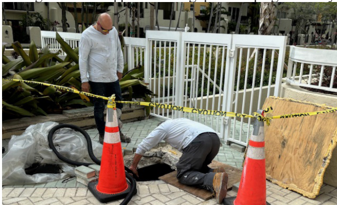
Deck Behind Social Room – Rainwater accumulation on lower concrete slab. Repair method is being developed. Estimated project completion: April 2024.
