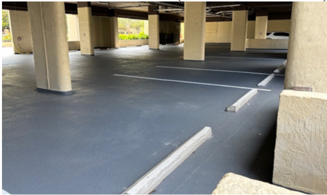
East Covered Parking - Waterproofing and traffic coatings have been applied. Parking spaces striping complete.
