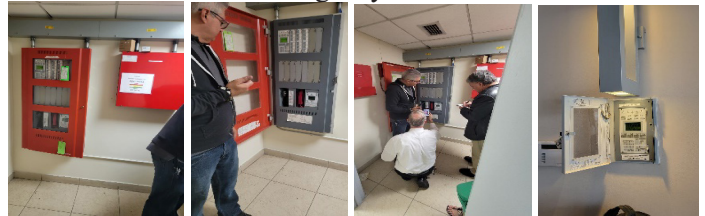
Fire panel located in the valet room.
