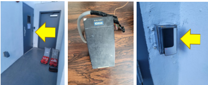
2 nd floor east side door fob reader (before & after)
