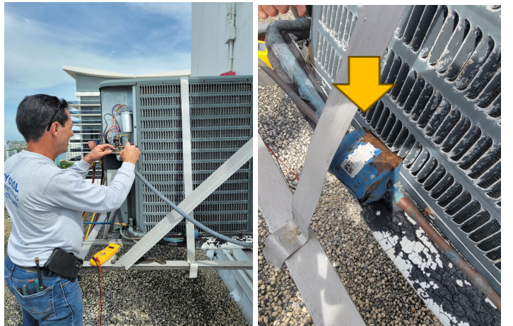
Faulty filter dryer
