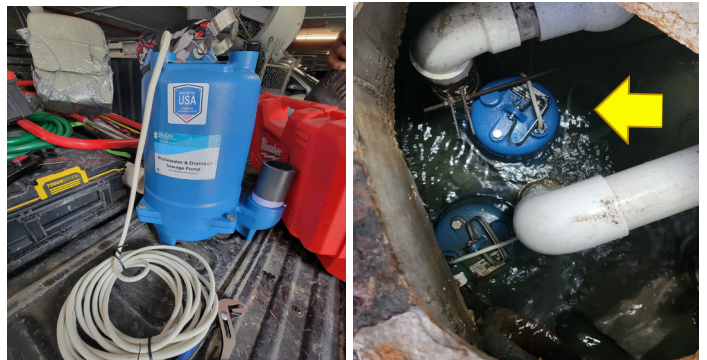
The 2 nd - New sump pump
