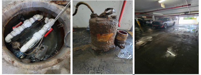
Old sump pump
