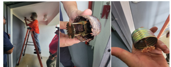
7 th floor old sprinkler head new sprinkler head
