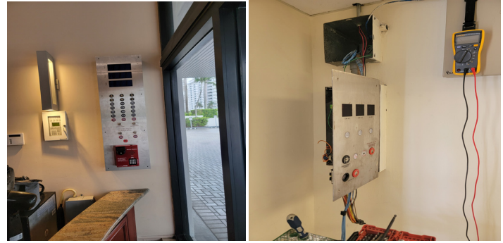
New elevator motoring system (old system)
