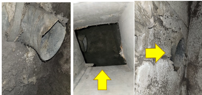
6 th floor dryer vent
