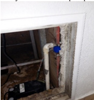
Maintenance cleaned the lobby a/c unit water pump.
